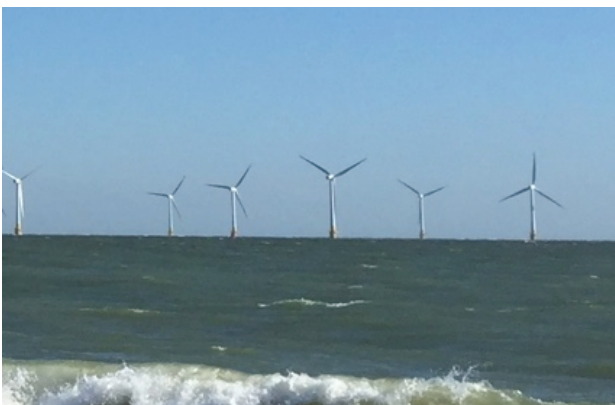
Offshore wind energy facilities in the U.K.
